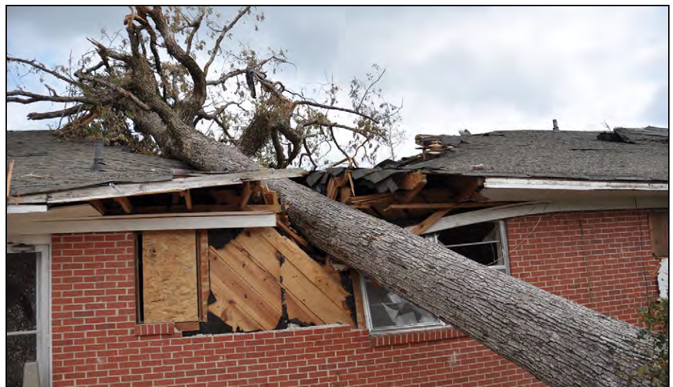
Figure B8-9. Large debris: Laydown of a large tree onto a nursing home. (Tuscaloosa, AL, 2011 tornado) (SOURCE: FEMA P-908, RECOVERY ADVISORY 6)
