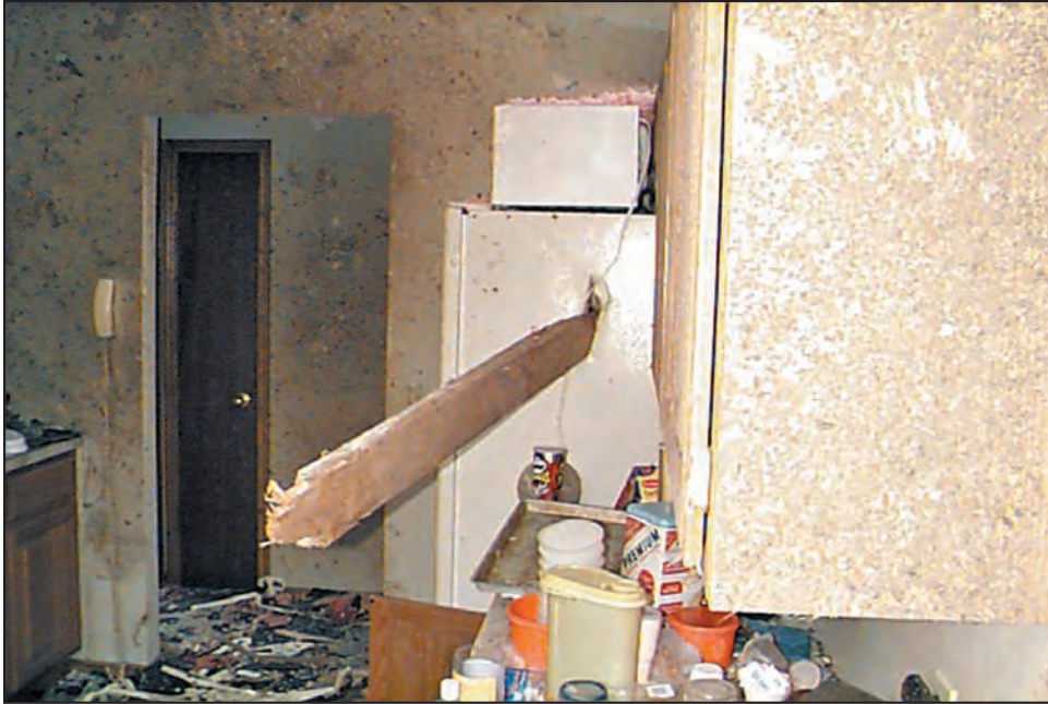
Figure B8-11. Refrigerator pierced by a 2x6. The portion of the 2x6 that is visible was 4 feet 8 inches long. It went several inches into the freezer compartment.
