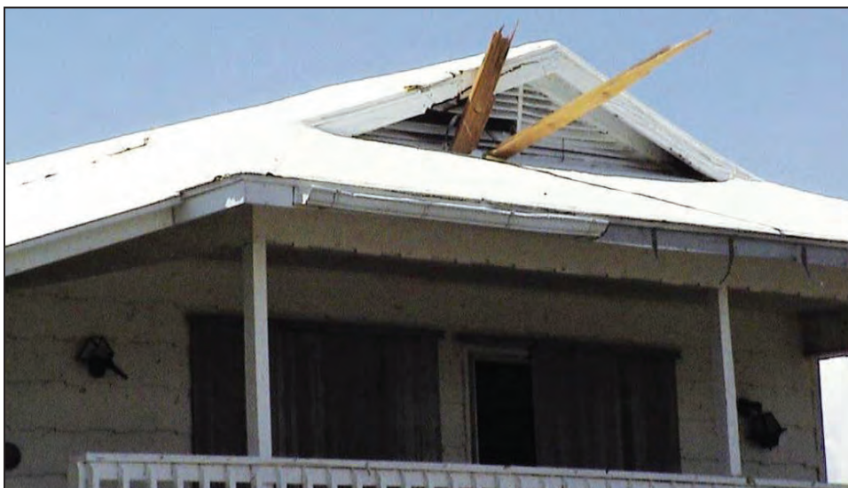
Figure B8-12. Impact of structural wood members in the gable end from a neighboring house (Pine Island, FL) (SOURCE: FEMA P-488)
