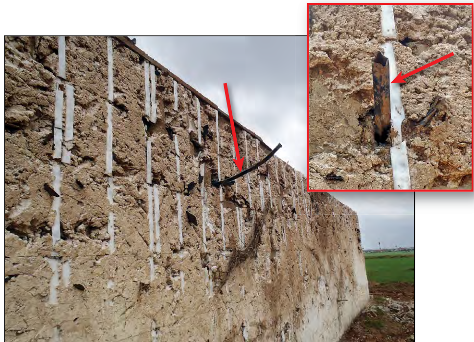
Figure B8 22. Red arrows show a steel tube that perforated a waffle grid ICF wall. Inset shows the tube in the “as found” condition and main photograph shows the tube after it was partially pulled out of the wall. (Moore, OK, 2013 tornado) (SOURCE: FEMA P-1020)
