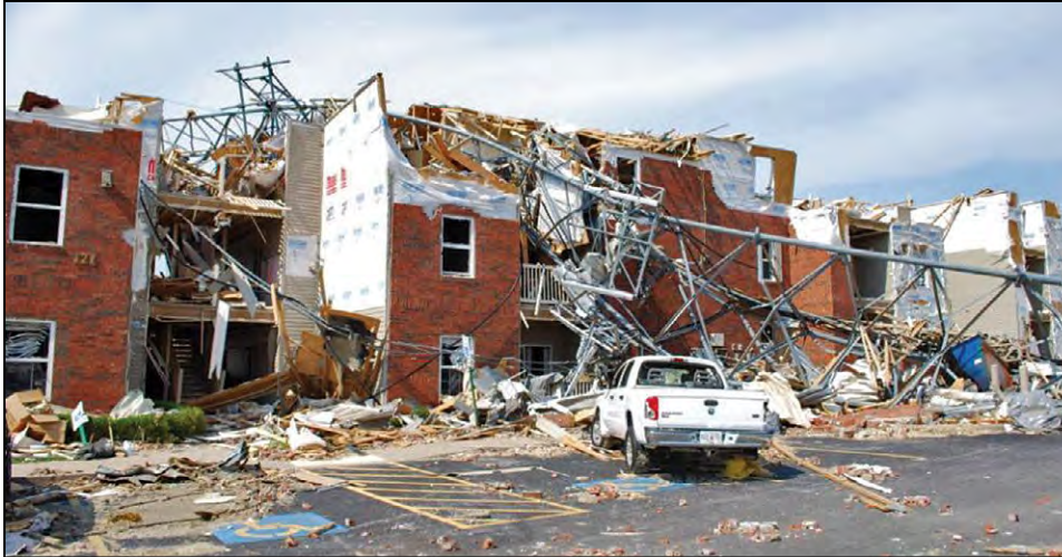
Figure B3-12. Lay down hazard: failure of a large communications tower onto a building (Joplin, MO, 2011 tornado)
