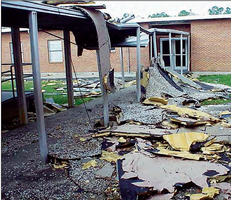
Figure B8-2. Medium debris: Pieces of a built-up roof from Hurricane Katrina (MS, 2005) (SOURCE: FEMA P-424)
