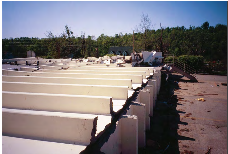
Figure B3-16. Collapse hazard: tall precast wall panels collapsed onto the floor slab (Midwest tornado, 2003)
