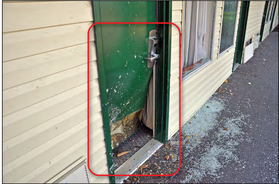
Figure B8-23. This metal door was damaged by wind-borne debris generated by a weak tornado. The bottom hinge was damaged, but the single latch was able to resist the modest wind and impact load. The door was on the verge of failing. (St. Louis, MO, 2013 tornado)
