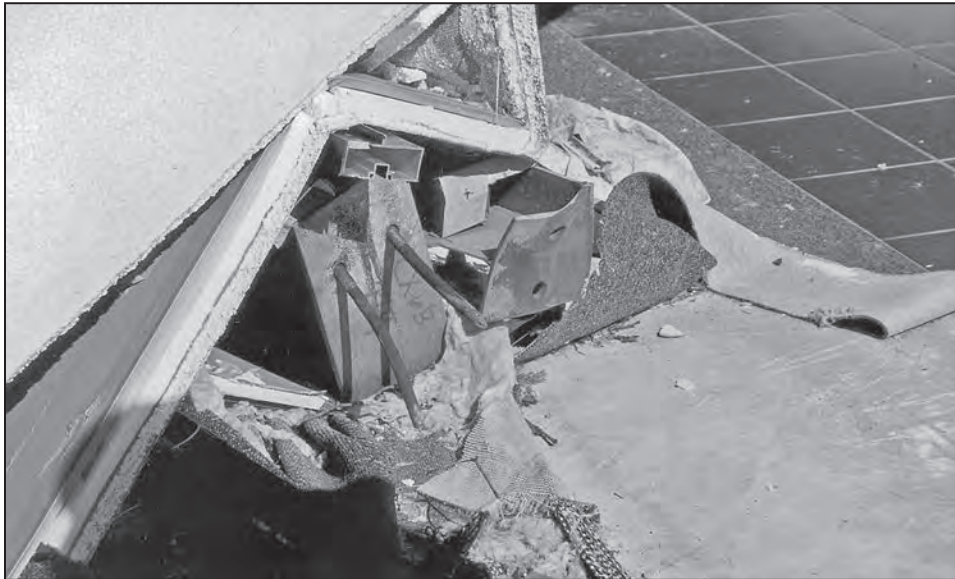
Figure B3-9. Two steel columns failed at their connection to the foundation when the anchor bolts that secured the column released from the concrete (embedment failure) while the anchor bolts that secured the column on the right experienced a ductile failure
