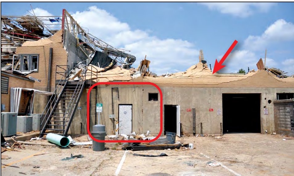
Figure B3-14. Collapse hazard: the story above an Emergency Operations Center collapsed. Masonry walls (red arrow) and part of the roof structure fell onto the second story floor slab above the EOC (Tuscaloosa, AL, 2011 tornado)
