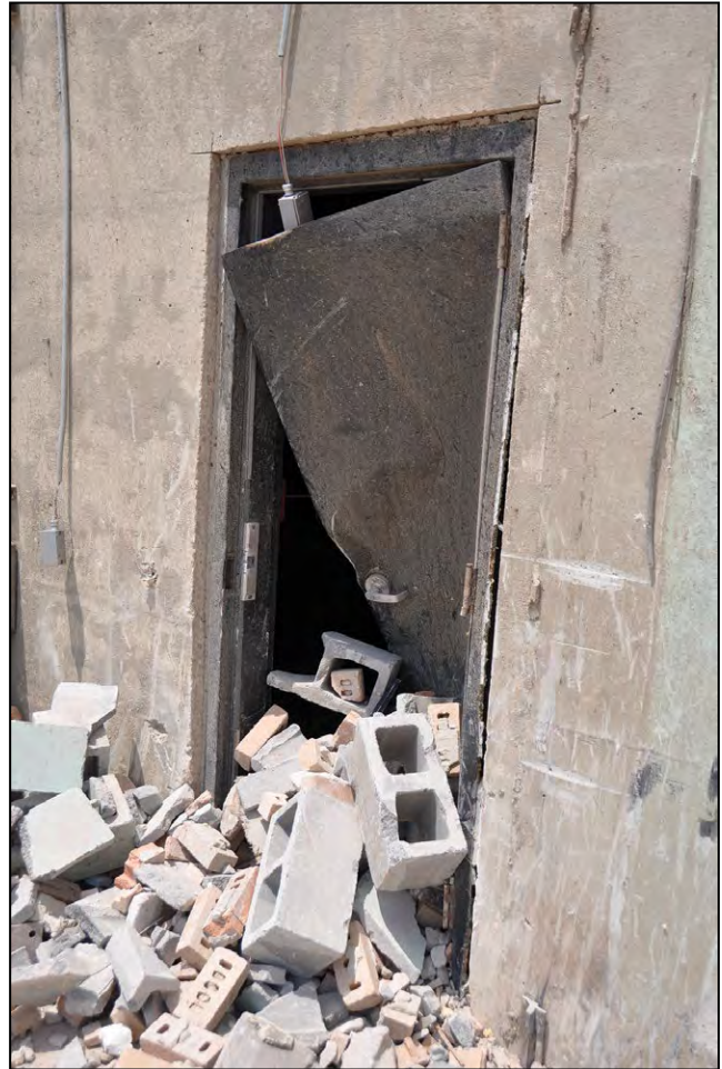
Figure B8-1. Metal door breached by wind-borne debris (this door was not designed to resist debris). (Tuscaloosa, AL, 2011 tornado)
