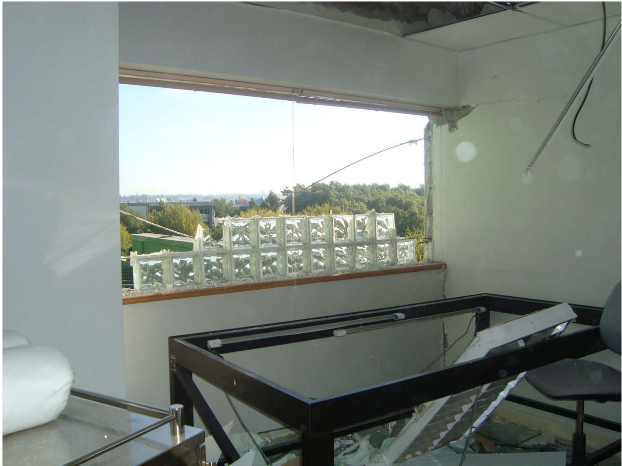
Figure 6.3.1.5-3 Damaged glass block panel from the Los Angeles Hospital in the 2010 Chile Earthquake; relatively new hospital building that had to be evacuated for repairs (Photo courtesy of Bill Holmes, Rutherford & Chekene). Blocks were installed with steel reinforcing bars in the top and bottom horizontal joints.
