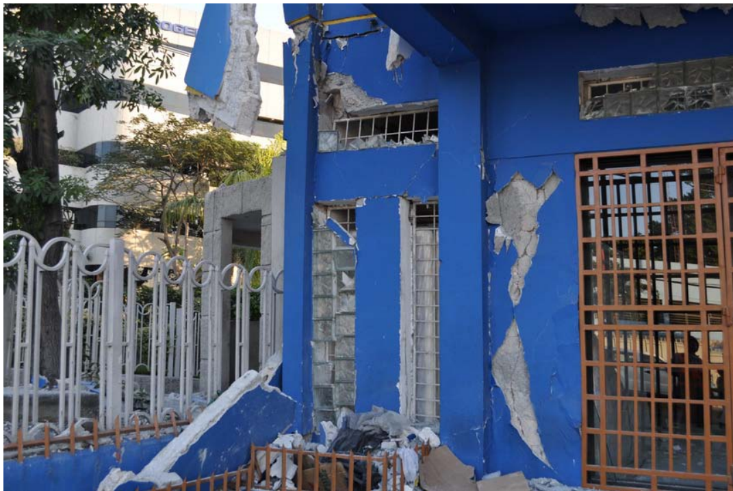
Figure 6.3.1.5-1 Damage to glass block in building with reinforced concrete frame and concrete masonry infill in the magnitude-7 2010 Haiti Earthquake (Photo courtesy of Eduardo Fierro, BFP Engineers). Note some blocks failed at rigid mortar joints and stayed in the frame, others fell out of the frame, and others broke in place. This building also suffered structural damage.
